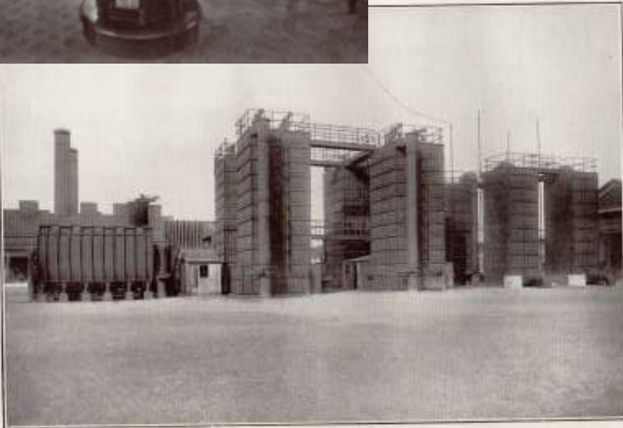
SCRUBBING AND WASHING PLANT.
